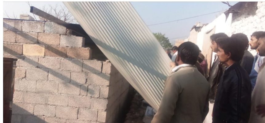
3 under construction boundary walls at Saidpur, 02 DPC, 02 rooms and a grill at Bari Imam. Encroachments at the roads of sector G-7 and G-8 have been
