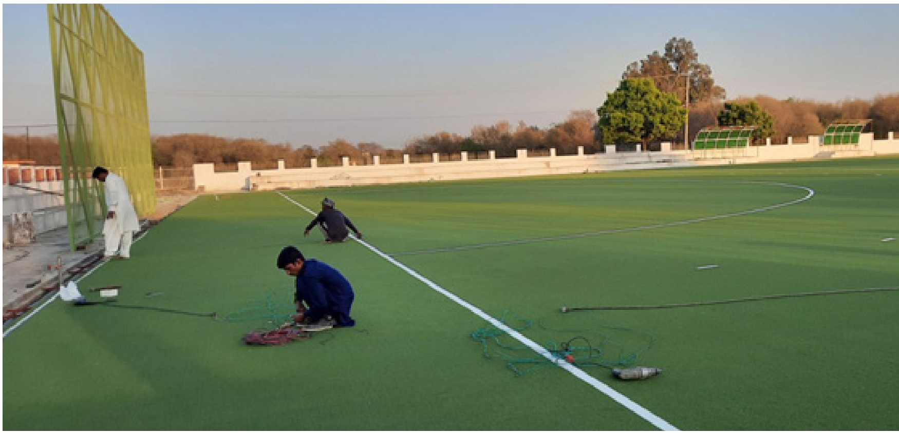
ISLAMABAD: Turf laying work at Naseer Bundha Hockey Stadium has almost been completed. The pitch shall be ready for use in one week after formal inauguration. – DNA
