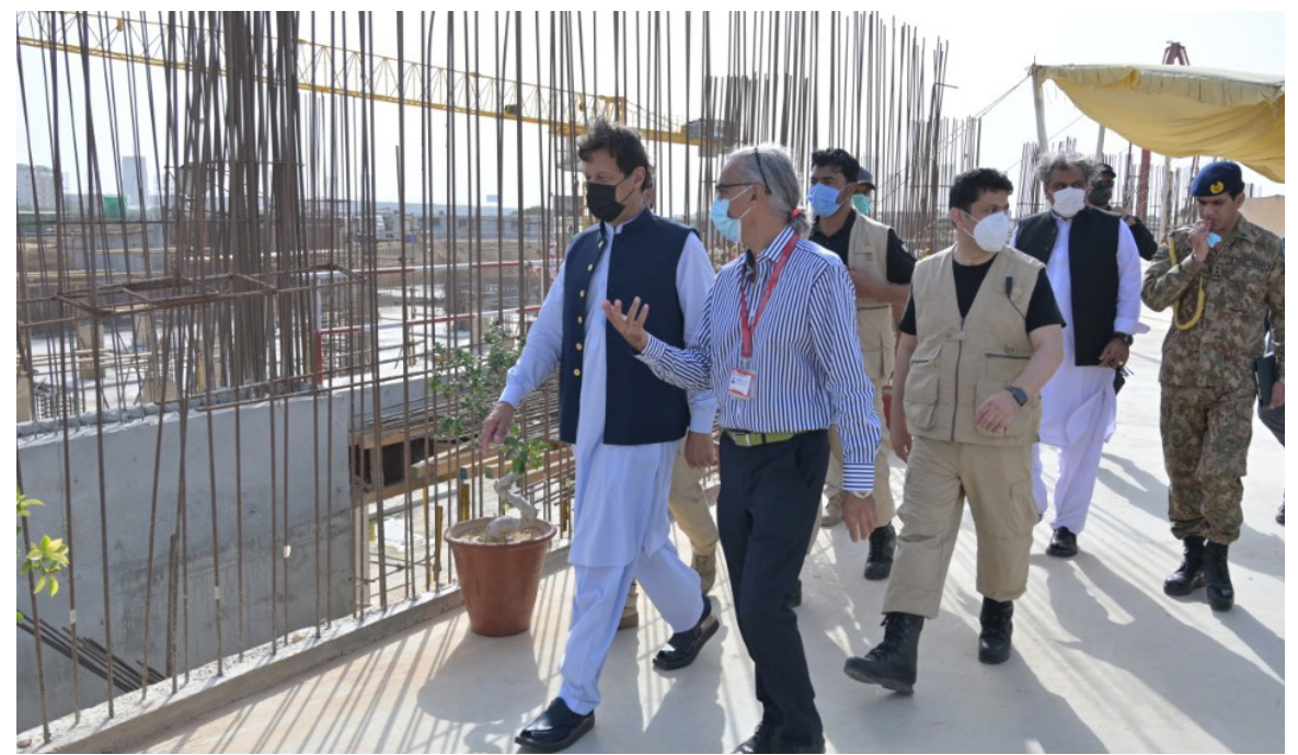
KARACHI: Prime Minister Imran Khan visits under construction Shaukat Khanum Memorial Cancer Hospital. – DNA
