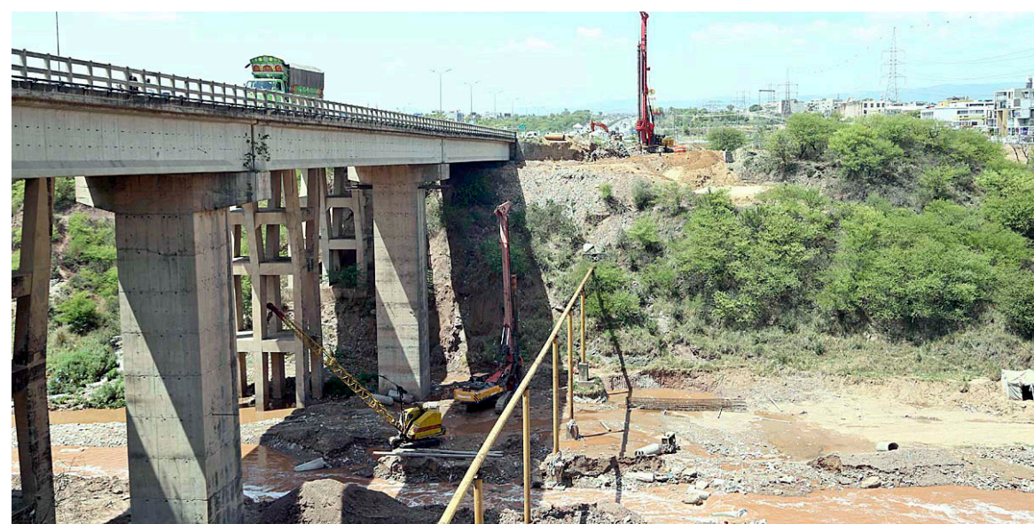
ISLAMABAD: A view of construction work of expansion of Expressway during development work in the city. - DNA
