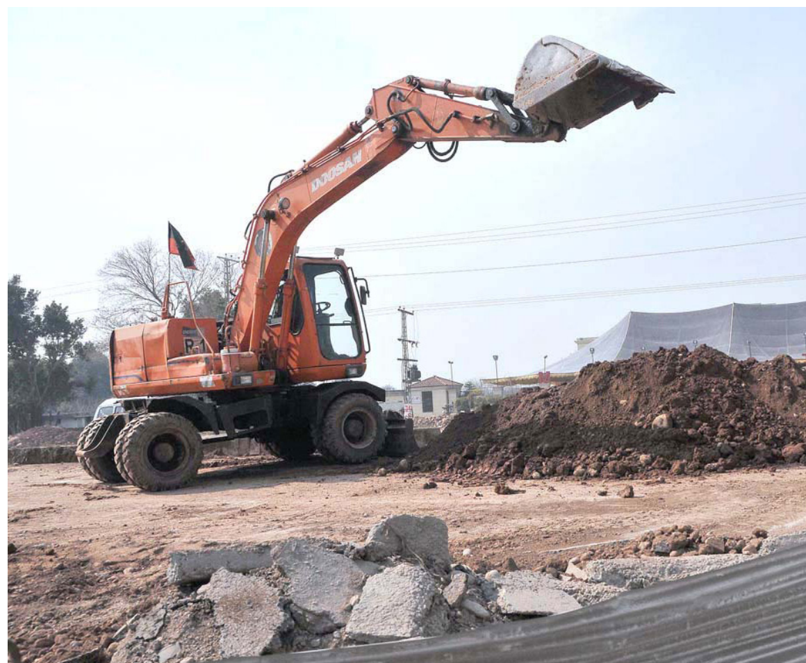
ISLAMABAD: A view of construction work of Rawal Dam Flyover underway during development work in Federal Capital. - APP
