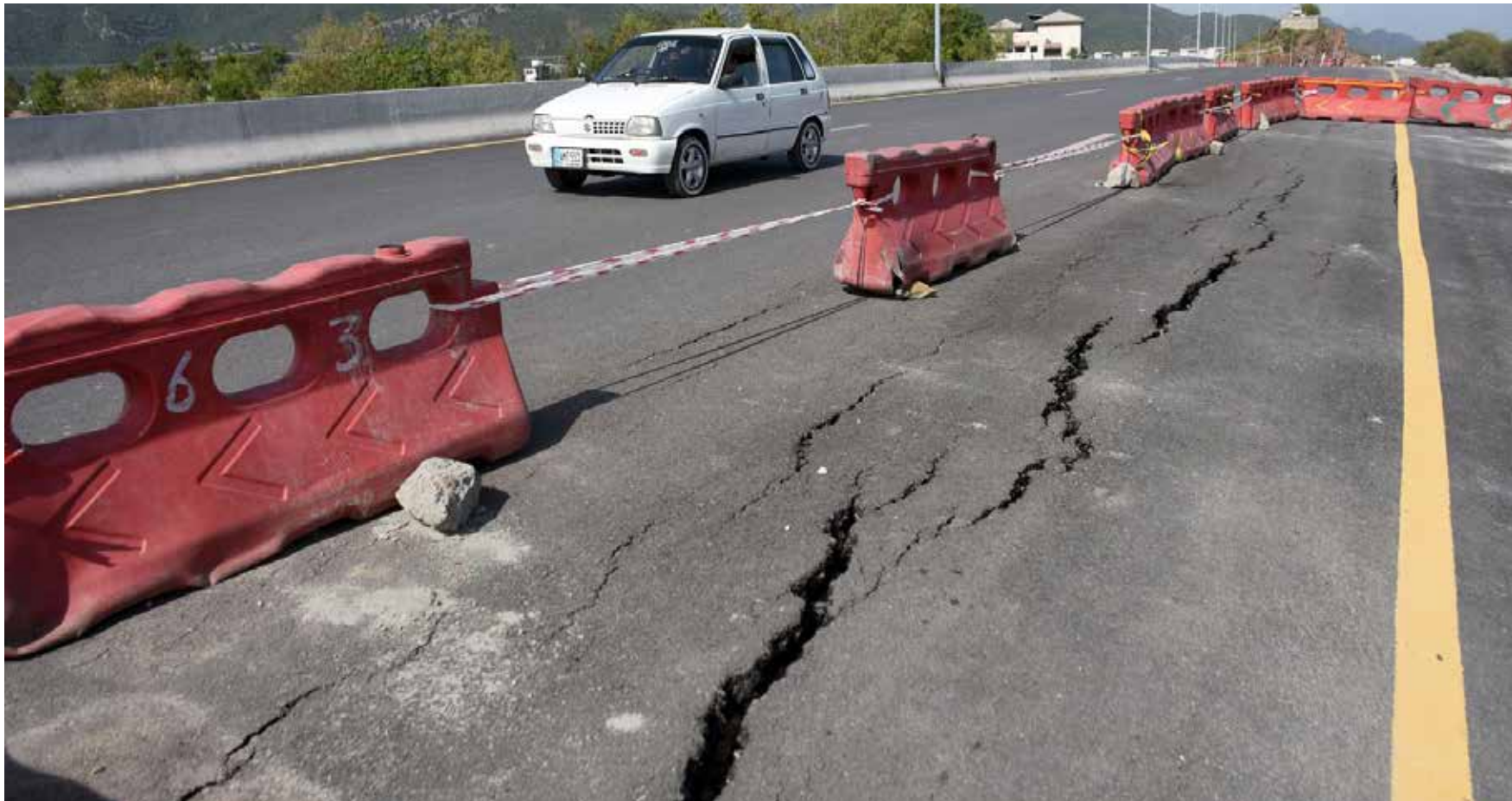
ISLAMABAD-April10: A view of cracks in the newly constructed Khayaban-e-Margalla Road as it is start destroying before opening properly for the traffic, which is the open sign of the usage of Low quality material during construction. —Online
