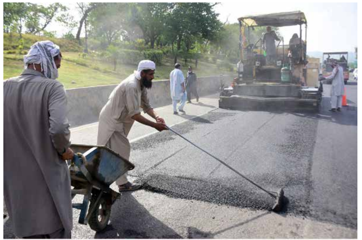
ISLAMABAD: Labourers are busy in carpeting the Faizabad Section of Express Way during high temperature in Federal Capital. —Online
