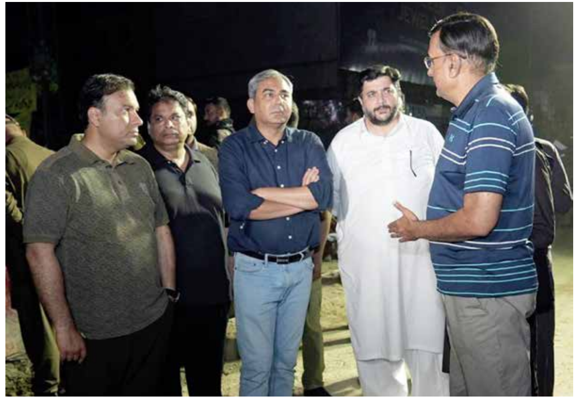
LAHORE: Caretaker Chief Minister Punjab Mohsin Naqvi inspecting the construction work on his visit to the under-construction Akbar Chowk flyover project.—DNA
