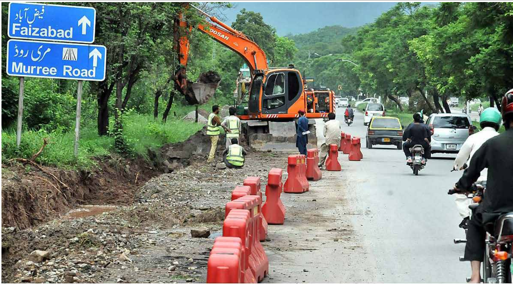
ISLAMABAD: During the expansion work of Club Road, heavy machinery is being utilized to carry out the construction and development tasks. —APP
