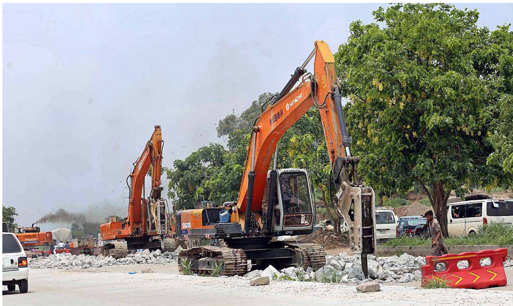
ISLAMABAD: August 07 – Heavy machinery being used for repairing the Islamabad Expressway during repairing work in Federal Capital.— APP
