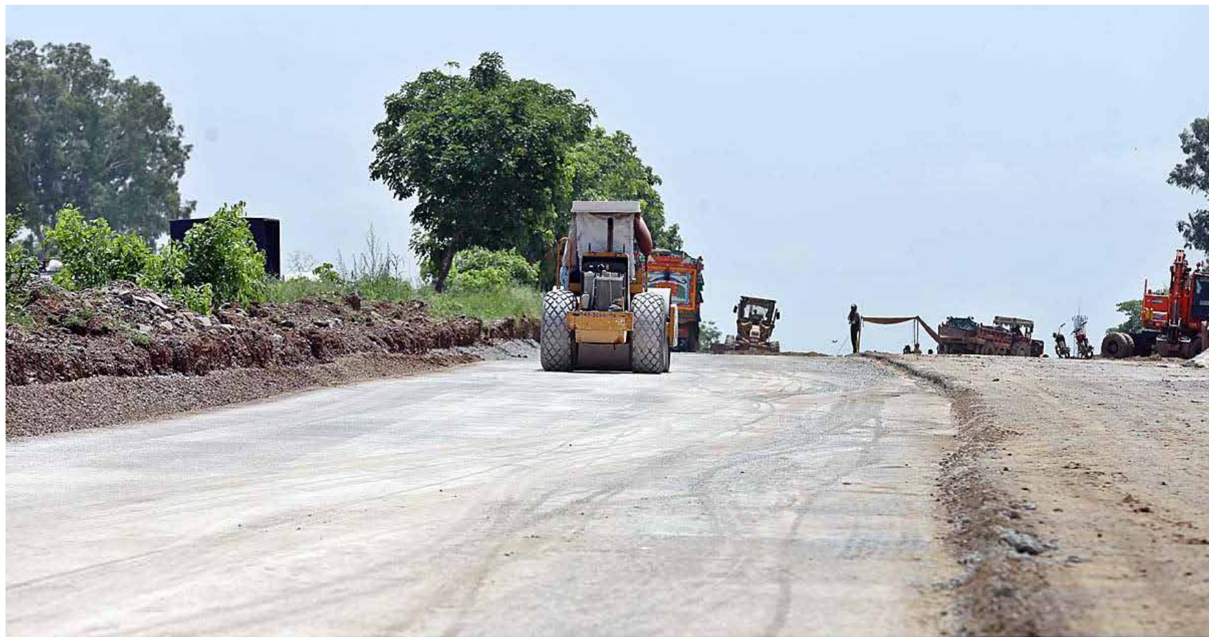
ISLAMABAD: Heavy machinery being used to expand a new lane on Islamabad Expressway. —APP
