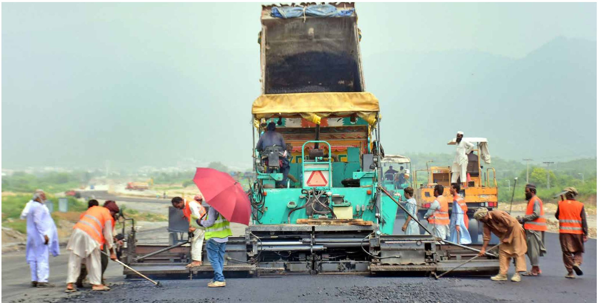
ISLAMABAD: Laborers are busy in carpeting of the road during the construction of E-11 Flyover in Federal Capital.—Online
