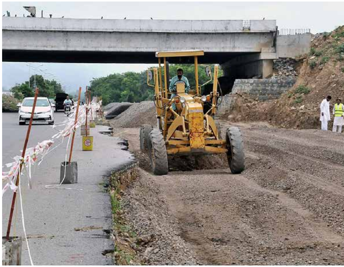
ISLAMABAD: Heavy machinery being used for construction work of Margalla Road during development work in Federal Capital.—APP
