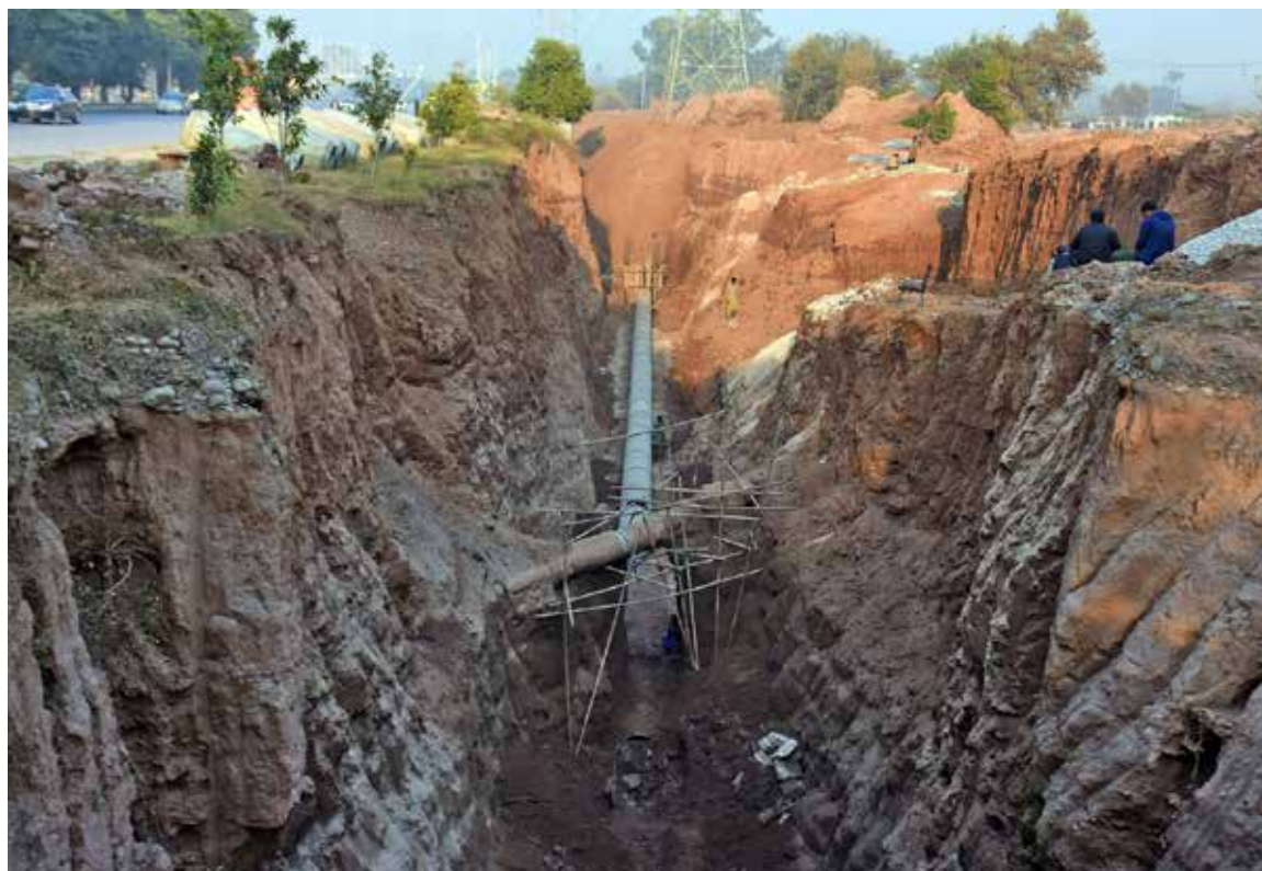
ISLAMABAD: A view of the under construction pipe line of the Rawal Interchange for evacuation rainy water after the several month of the completion of under pass, which needs the investigation by high authorities to find out the suspect of wasting tax spares money of the nation.—ONLINE
