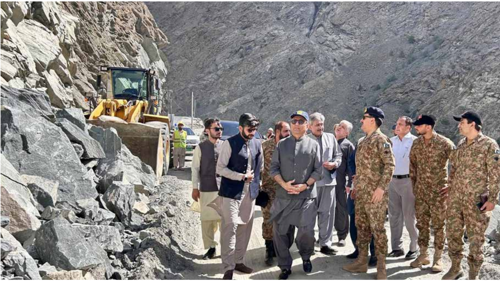
Federal Minister for Communications, Privatization & Board of Investment, Abdul Aleem Khan inspecting land slide in Skardu on May 6, 2024.
