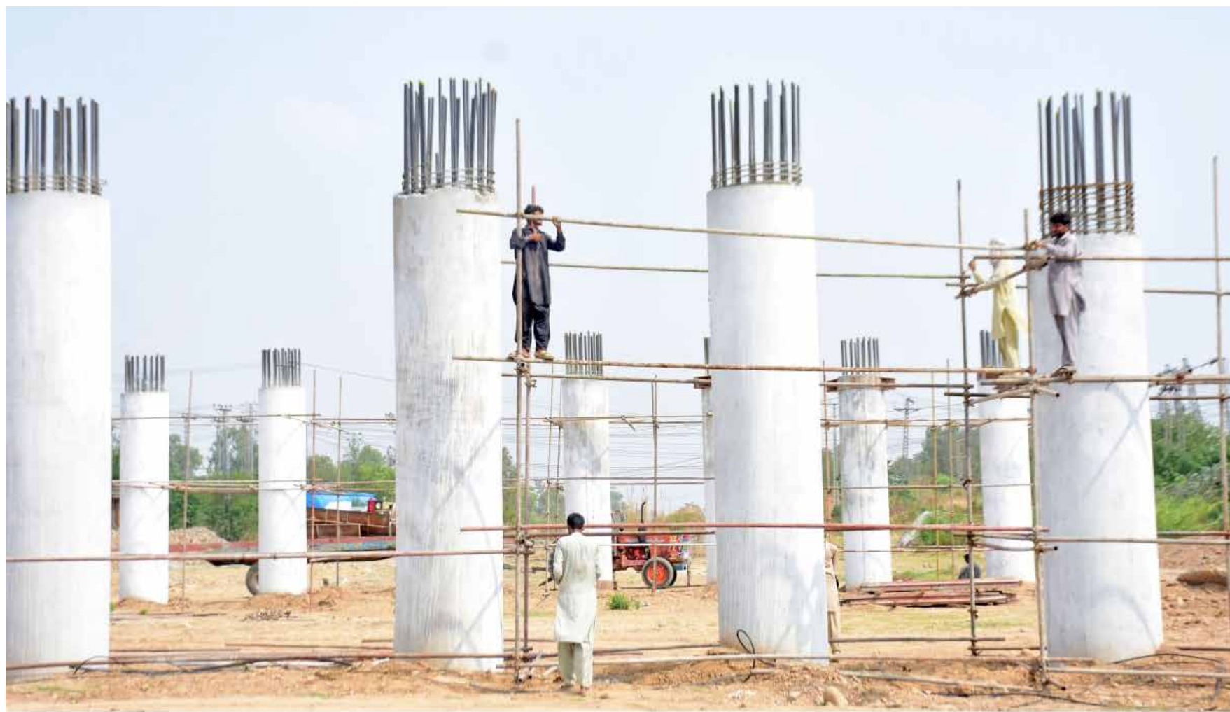
ISLAMABAD: Work continue on the construction project of an Overhead bridge at Sector 1-10 for connecting Sector H-10 to 1-10 and onwards with Margallah Avenue in the Federal Capital.— ONLINE
