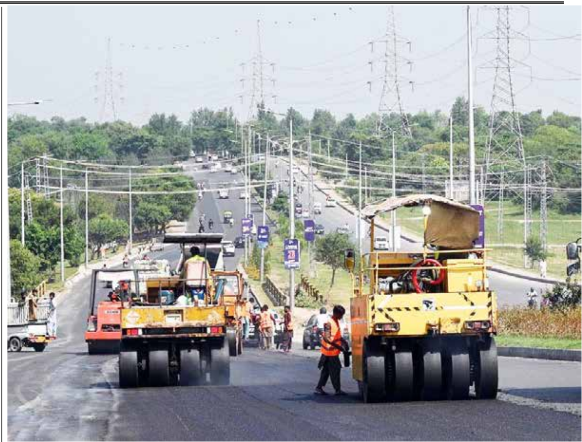
ISLAMABAD: Labourers busy in road construction with the help of heavy machinery during development work near Faizabad.—APP
