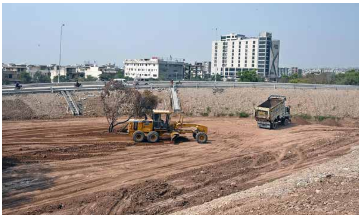
ISLAMABAD: Machinery is being used for leveling the ground to prepare a green area along the road near Kakpul. APP
