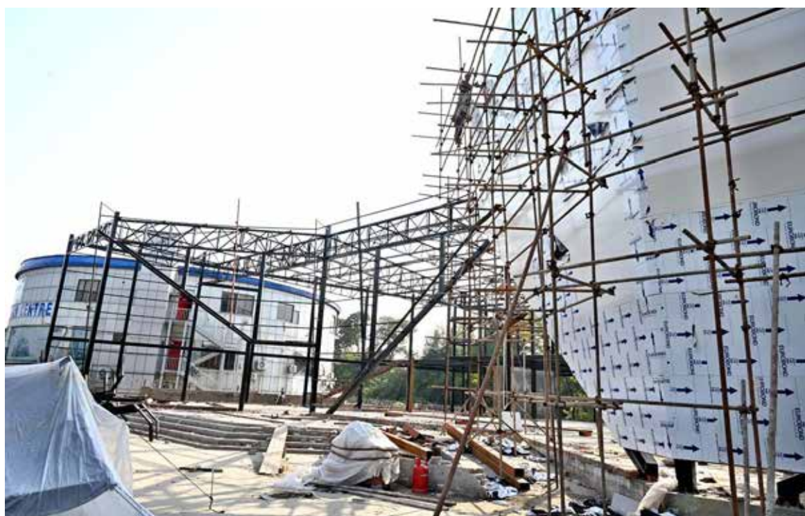
ISLAMABAD: Labourers busy in construction work of CDA Business Facilitation Centre at G-7 sector.—APP
