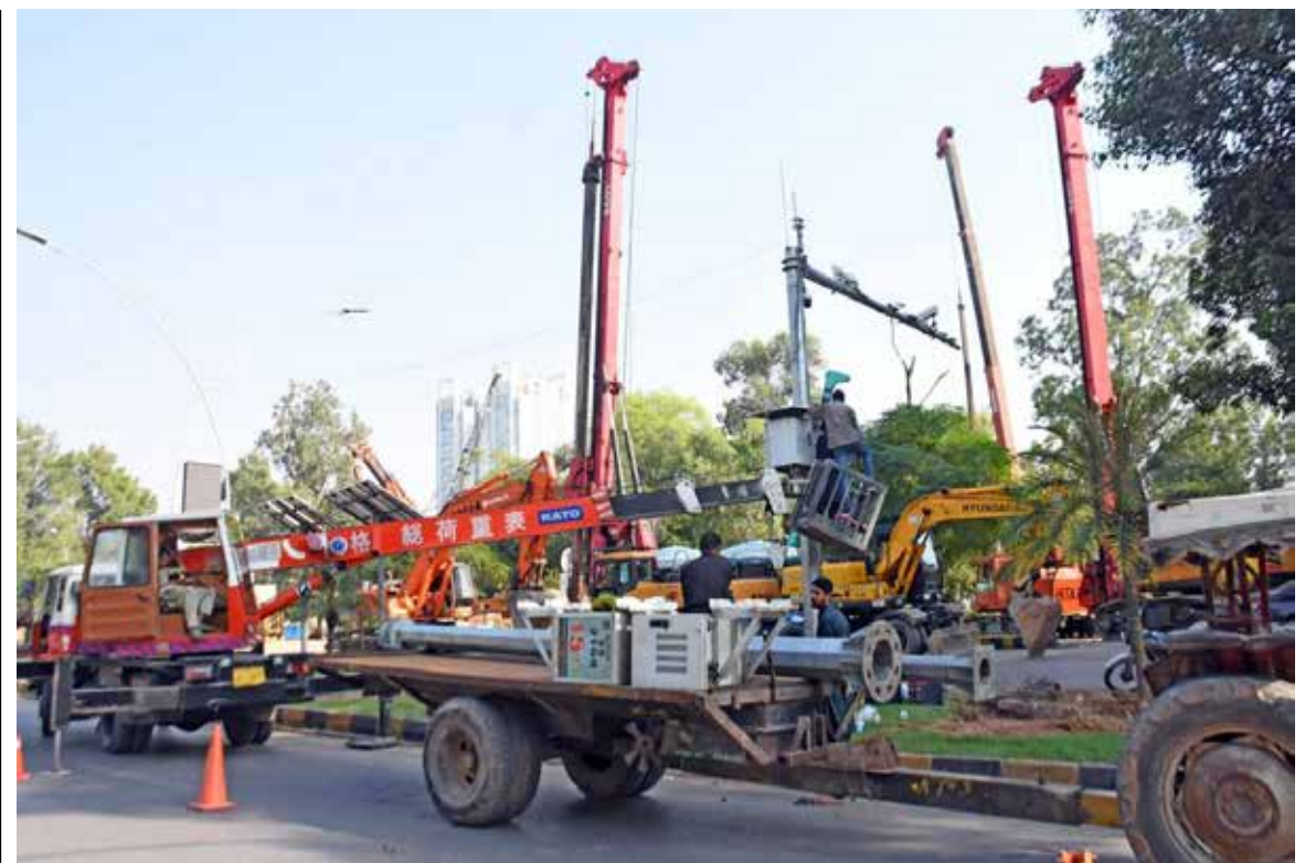
ISLAMABAD: Safe City cameras being take off owing to the Construction of Underpass at Khayaban-e-Suhrwardy Road.
