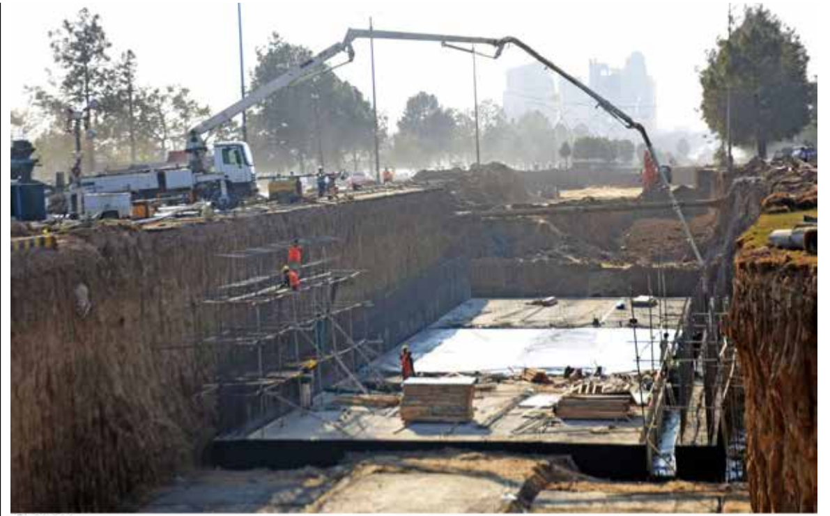
ISLAMABAD: Construction work on Jinnah Avenue flyover and underpass simultaneously kicked off in the Federal Capital.
