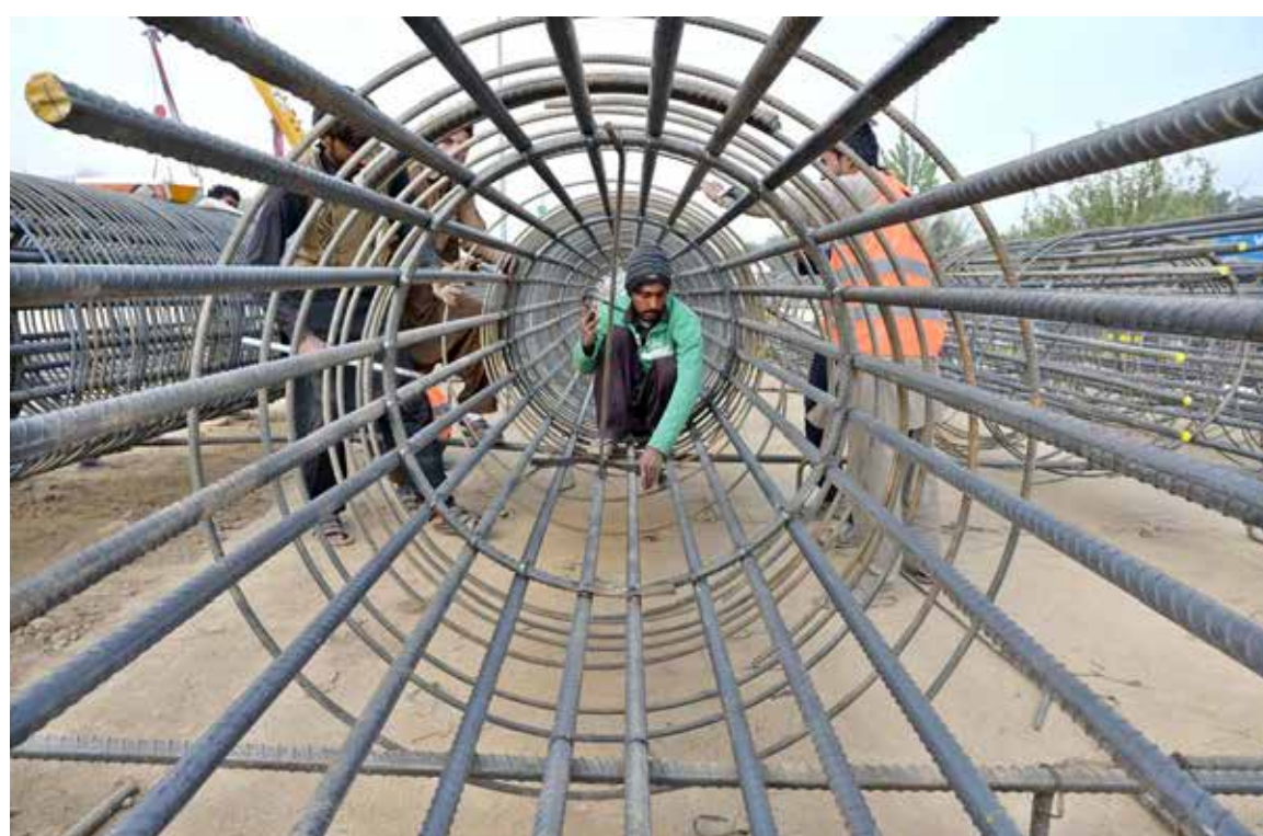
ISLAMABAD: Labourers are busy in work at the site of under-construction PTCL Chowk underpass project during development work in Federal Capital.
