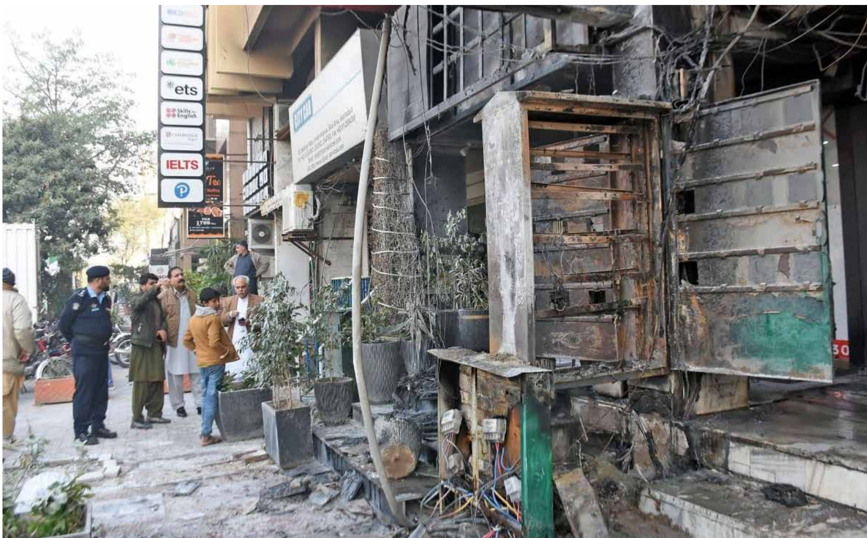
ISLAMABAD: Burned shops due to short circuit at Shalimar Plaza blue area, in the Federal Capital.
