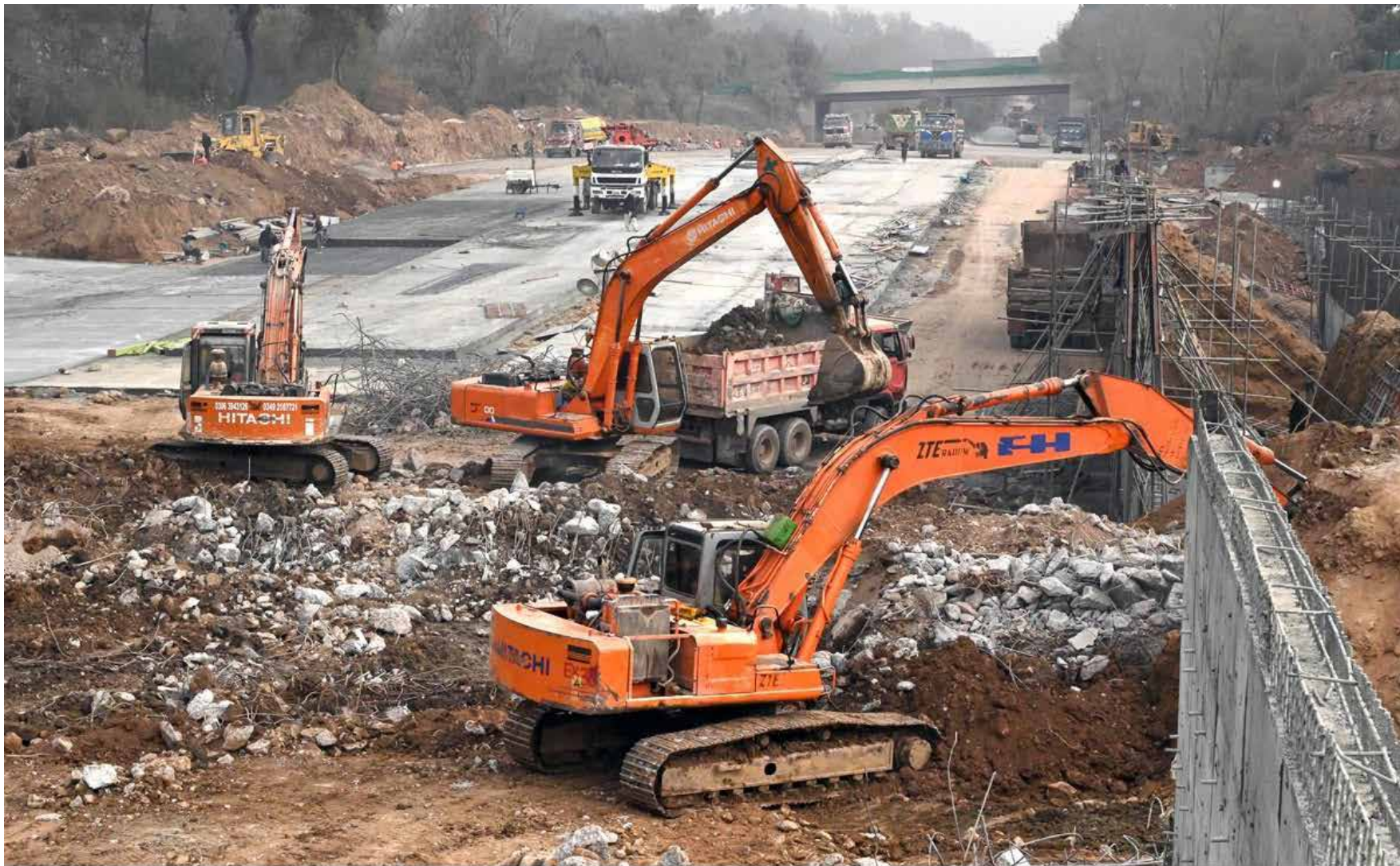
ISLAMABAD: Heavy machinery being used for construction work of Serena Chowk Underpass Project during development work in Federal Capital.
