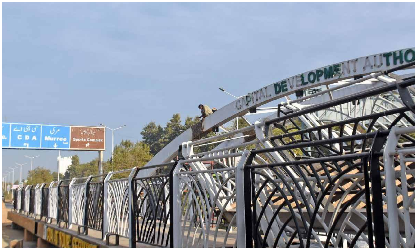
ISLAMABAD: A worker busy in welding of a pedestrian bridge as installing at Srinagar Highway in front of Rose & Jasmine garden, in Federal capital.
