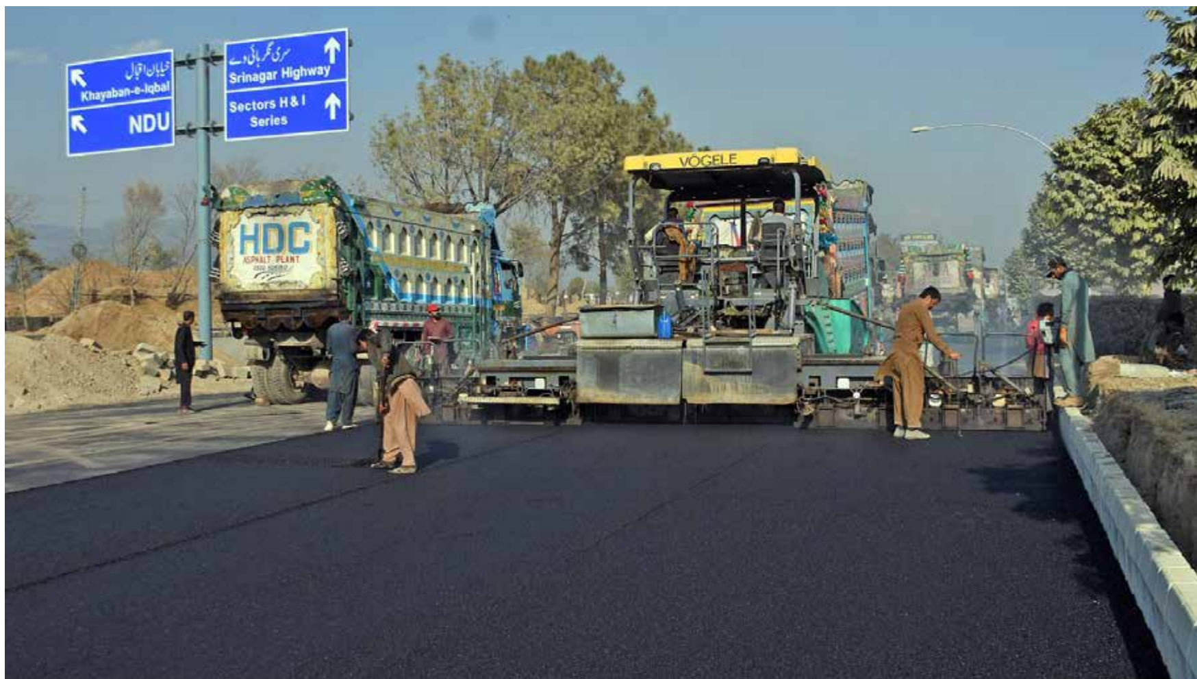
ISLAMABAD: Labourers busy in carpeting on a newly constructed road during of F-8 Exchange Chowk Interchange project during development work, in Federal Capital.
