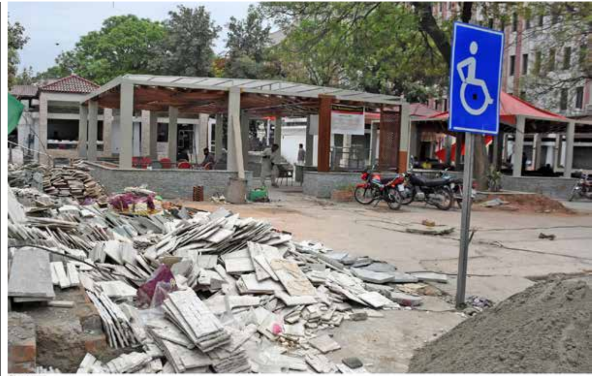
ISLAMABAD: Construction work at Melody Food Park continues at very slow pace, needs attention of authorities concerned.
