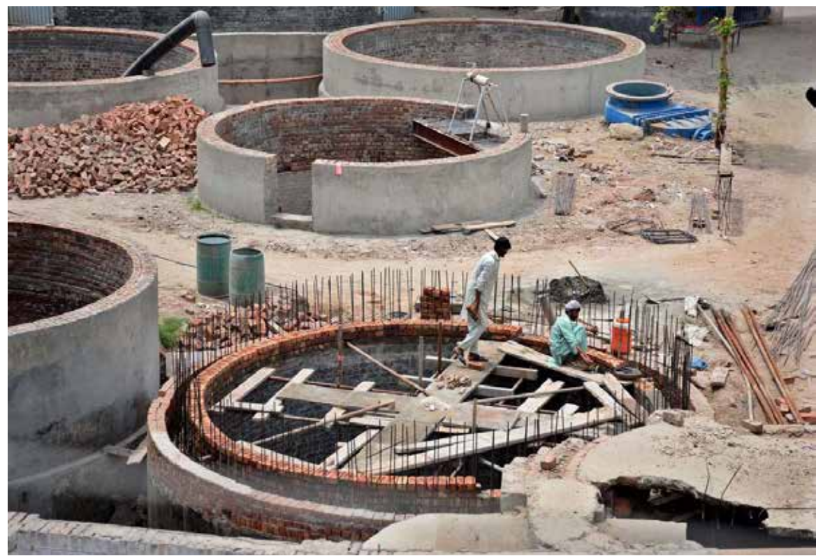
MULTAN: Labourers busy in the construction of a sewage disposal system at Chungi No. 9 as part of an ongoing development project to improve civic infrastructure in the city.
