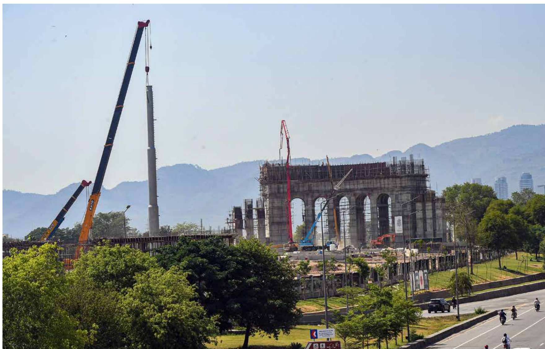
ISLAMABAD: A large crane hoists a towering flagpole into position at the construction site of the "Marka-e-Haq Monument, as work on the grand structure progresses rapidly, with the scenic Margalla Hills forming a striking backdrop.
