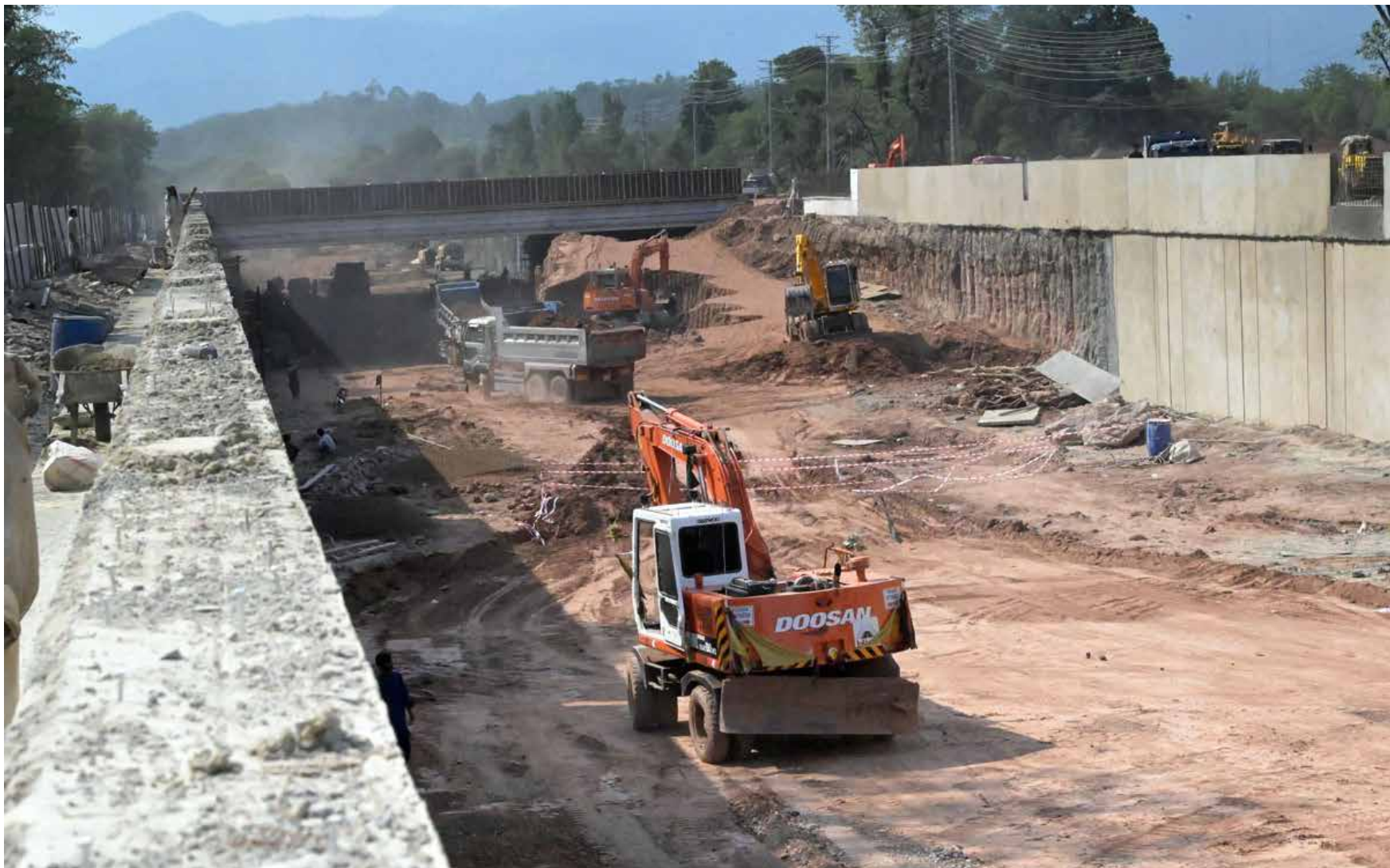
ISLAMABAD: Heavy machinery being used in construction work at the Park Road underpass project in the Federal capital.
