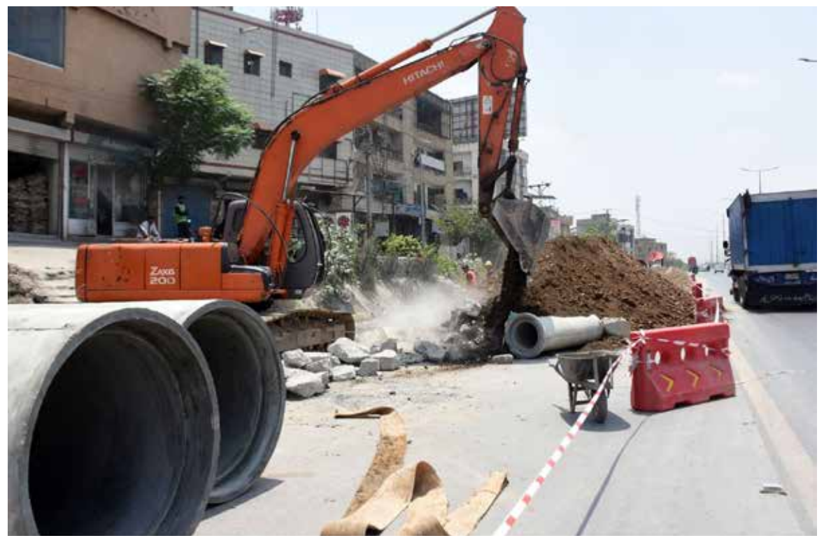
ISLAMABAD: Workers busy in digging with heavy machinery for installing new sewerage line at Karnal Sher Khan Shaheed Road, during development work, in the Federal Capital.
