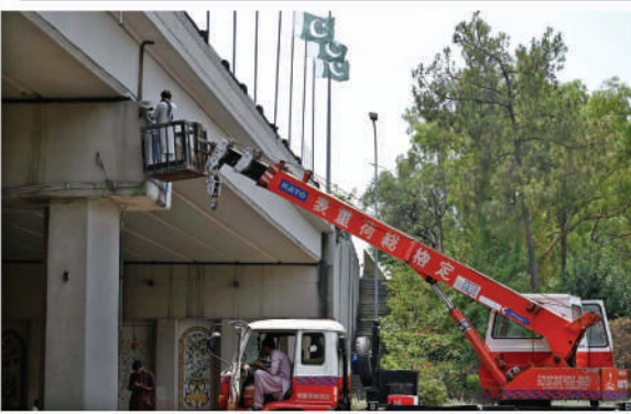
ISLAMABAD: A worker busy installing CCTV camera for safety purpose on bridge near zero point
